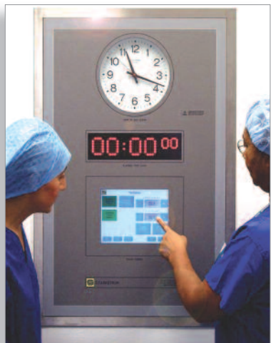
Theatre Control Panel
